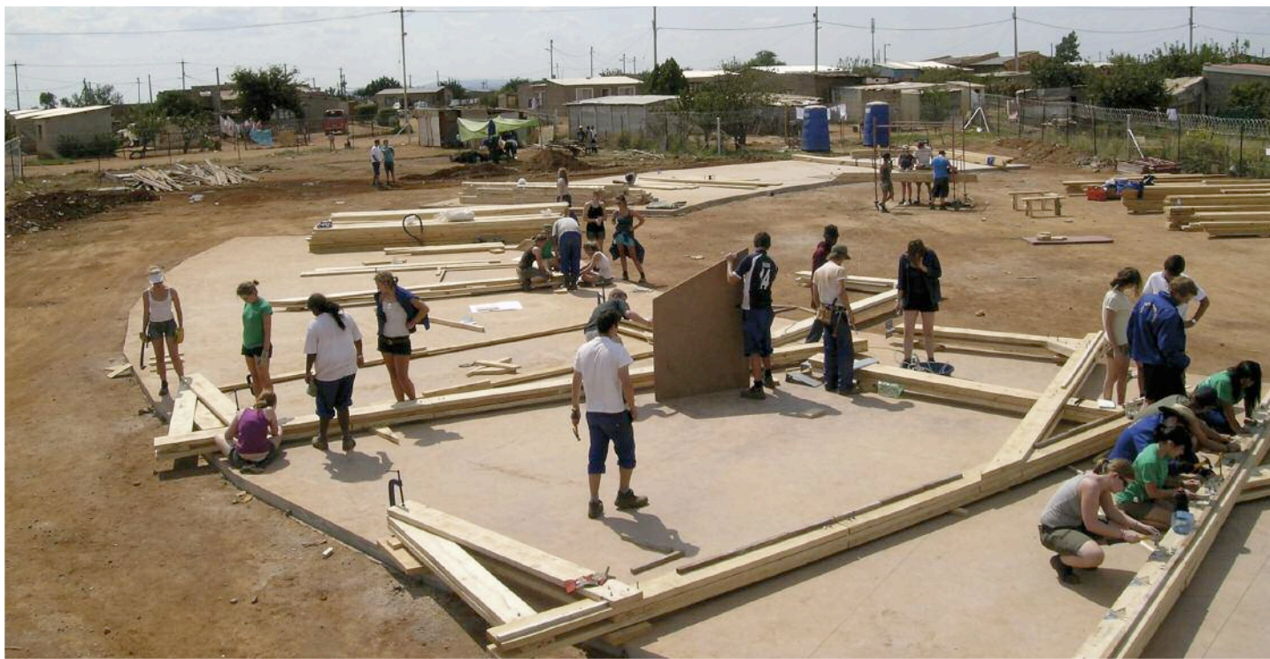
Left: Setting out the trusses in week three. Students on the far right fix hurricane joist clips
